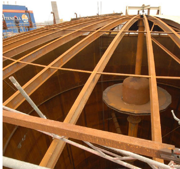
Figure 3. Upper orifice in the TES tank in CHP Siekierki-Warsaw [28].
